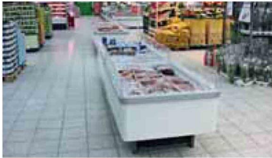
Measuring chests with condensers clogged with different levels of dirt.
