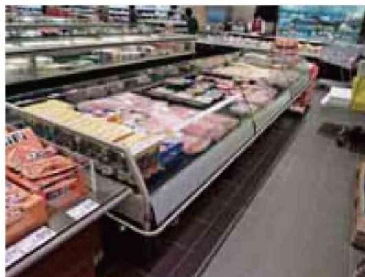
Figure 59: MT island 1, refrigeration zone
