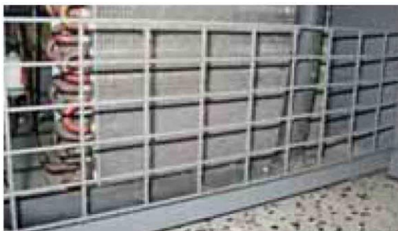
Moderately dirty condenser – power consumption +10%.
