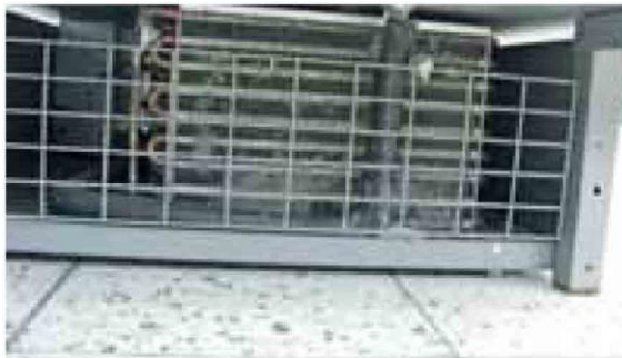
Condenser clean or with almost not dirt – basis power consumption 100%.
