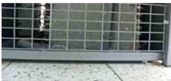
Very dirty condenser – power consumption +15%.
