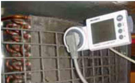
Figure 49: Dirt on the condenser 1
